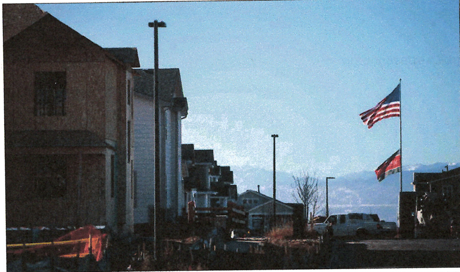
Houses in various states of construction can be seen Dec. 12 in the Aurora Highlands Metro District in Aurora. TIMOTHY HURST, THE DENVER GAZETTE
